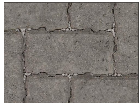
Image1 Permeable block paving
